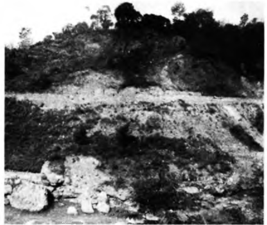
Fig. 2: Panoramic view of Narayanbagar landslide showing toe erosion of slope
